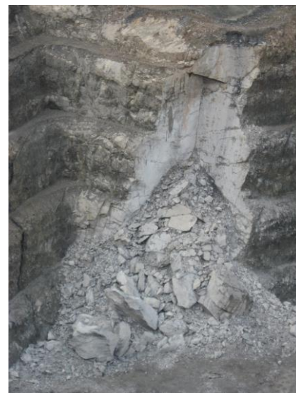
Figure 1 Wedge failure on a bullnose
