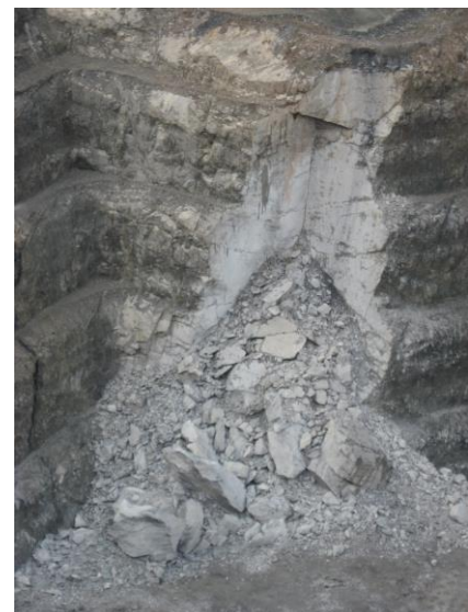
Figure 1 Wedge failure on a bullnose
